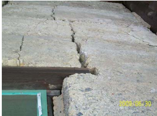
Figure 8: The crack and cavity at lintel end
