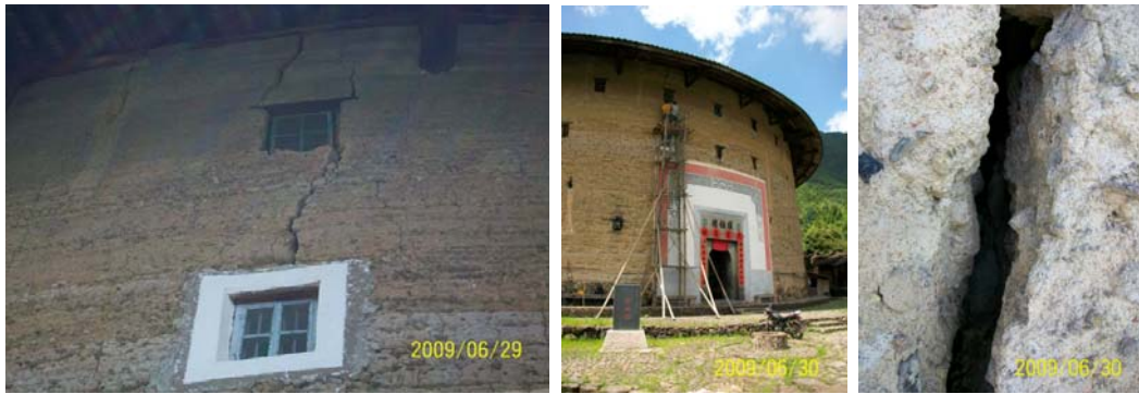
Figure 7: Huanji Tulou wall crack after earthquake, a) a global view of the crack, b) the crack location with reference to the ground and the access platform used during field study, c) close view of the crack
