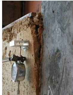
Fig. 6 Failure of W3
