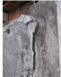
Fig. 7 Failure of reinforced wall
