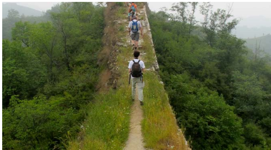
Slip section with Rammed Earth Core torn and exposed at an angle. #5
