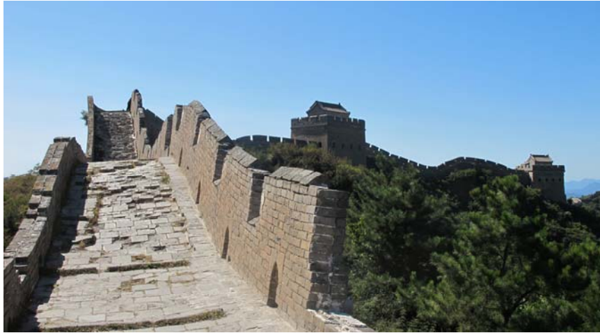
Figure 11. Outward lean. Parapet on right fallen away. #4
