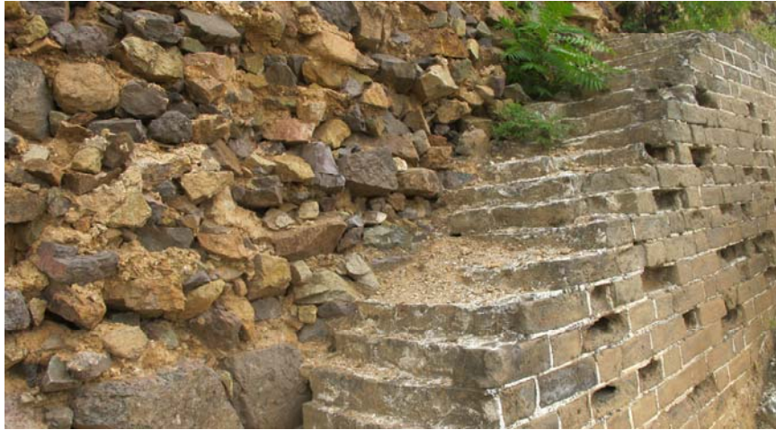
Figure 8. Rubble Core. Brick wall leaning in. #5
