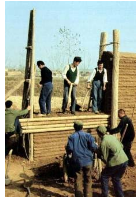
New rammed earth wall, Xi'an. Courtesy of Satprem Maini, Auroville Earth Institute
