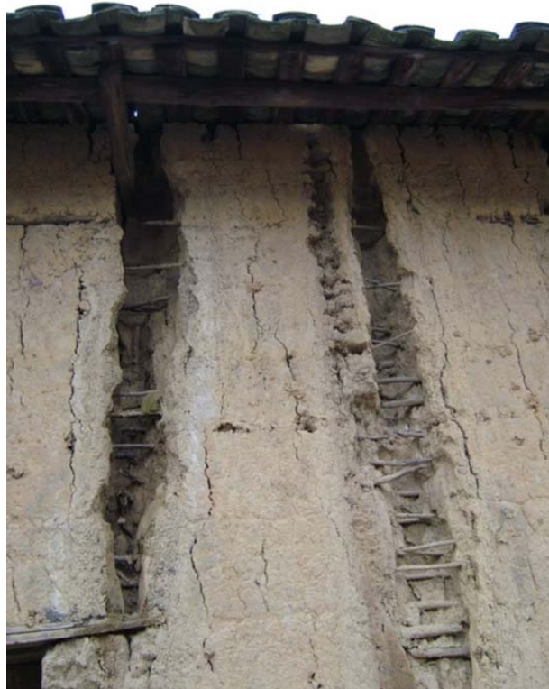
Eroded RE wall exposing wall ribs
