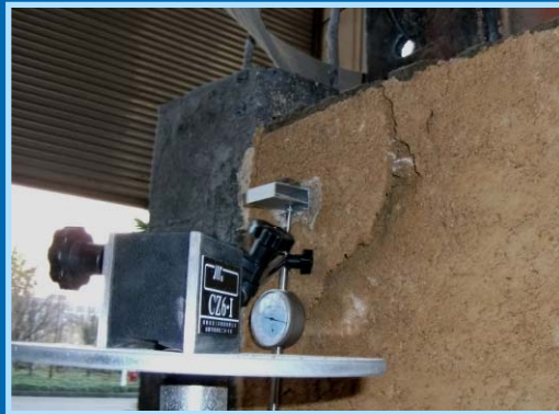
Crack in the upper boundary
