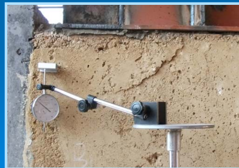
Cracks on both sides of the upper corner
