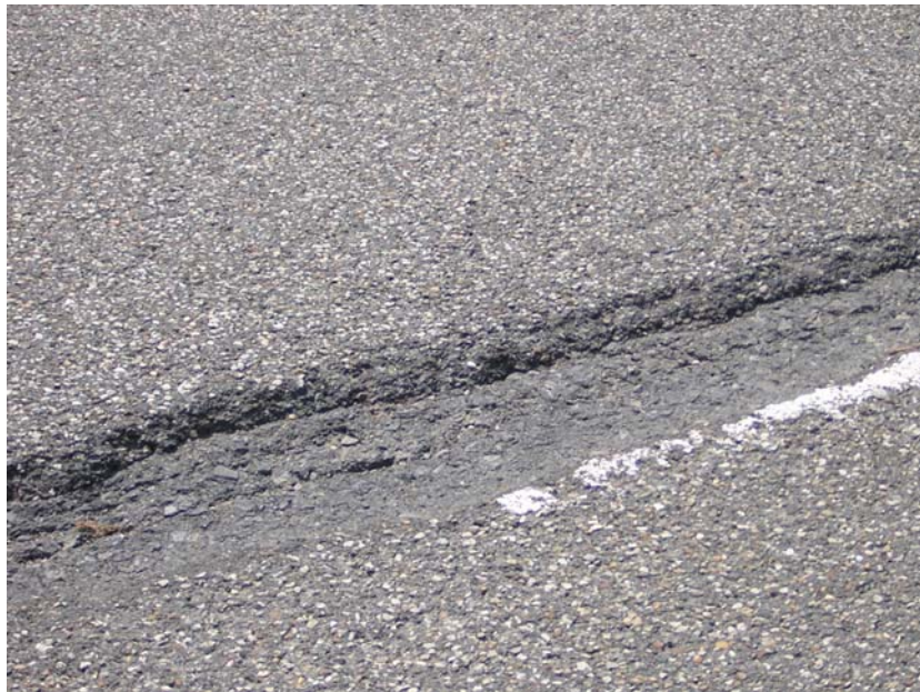
Figure 1.1 Failed pavement on I-68 in West Virginia
